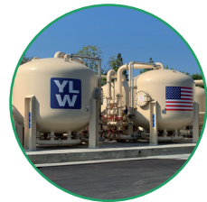
PFAS treatment plant for drinking water by Tetra Tech, using reverse osmosis and nanofiltration.
